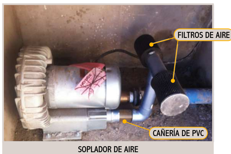
Figura 33: Blower Baldor 5 HP
